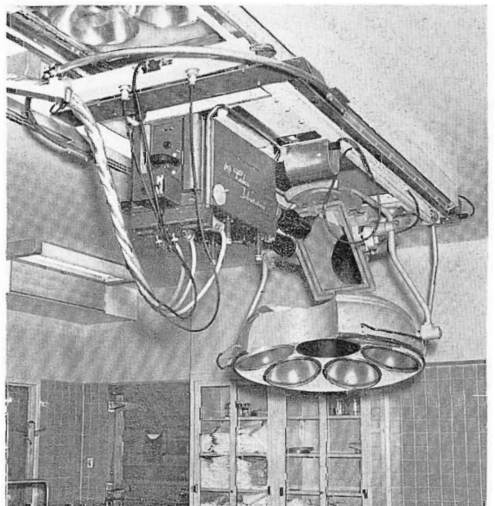
FIG. 11. Ceiling-mounted camera can be swung through full 360 degrees. Travel in north-south and east-west direction controlled by wall switches.
