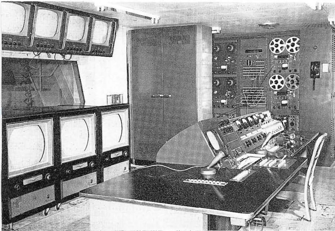
FIG. 3. Master control at AFIP. Programs from all three buildings are received and distributed from here. Window at left overlooks main studio.
