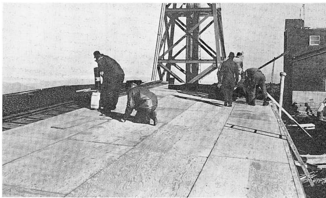
FIG. 16. Prefabricated plywood panels are set in place in the first stage of reinforcing the transmitter house roof.
