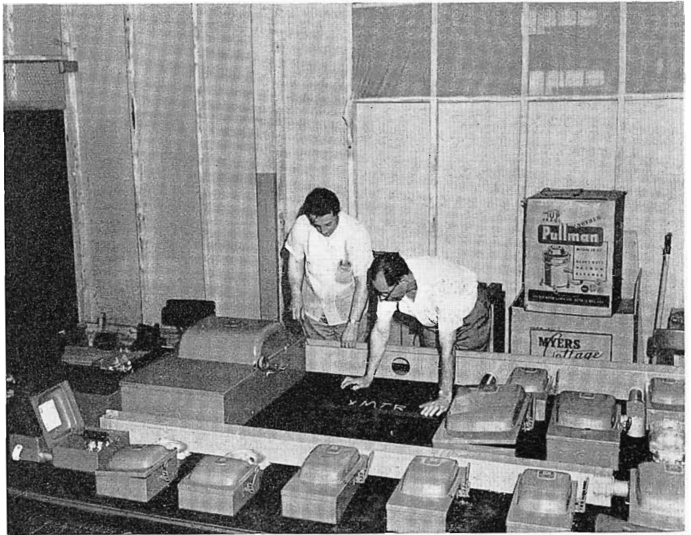
FIG. 12. Power load center is carefully laid out and preassembled. Other units usually assembled on the job, such as water systems and air ducts, were also prefabricated.
